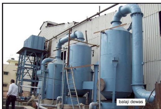
FOUR STAGE VENTURY AND SCRUBING SYSTEM
