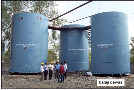
ACID STORAGE TANK
