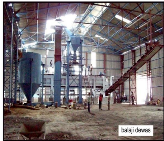
FULL VIEW OF S.S.P PLANT
