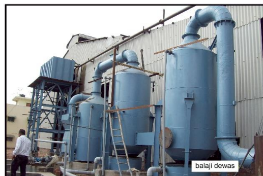
FOUR STAGE VENTURY AND SCRUBING SYSTEM
